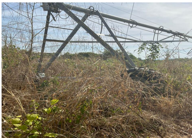
Figure 16: Shikabeta Irrigation Scheme's Centre Pivot submerged in dense vegetation.
